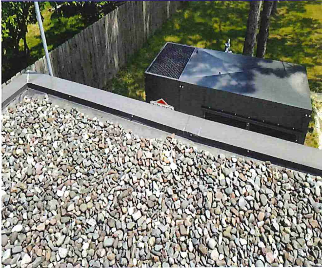
Minor bridging around the entire perimeter.
