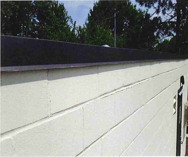
6' crack in the block wall.
