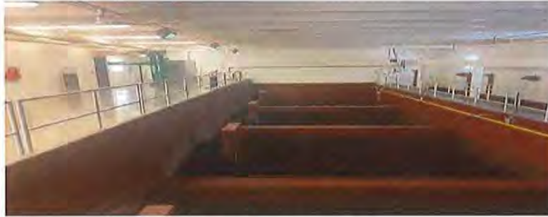
Water Treatment Facility Filters
