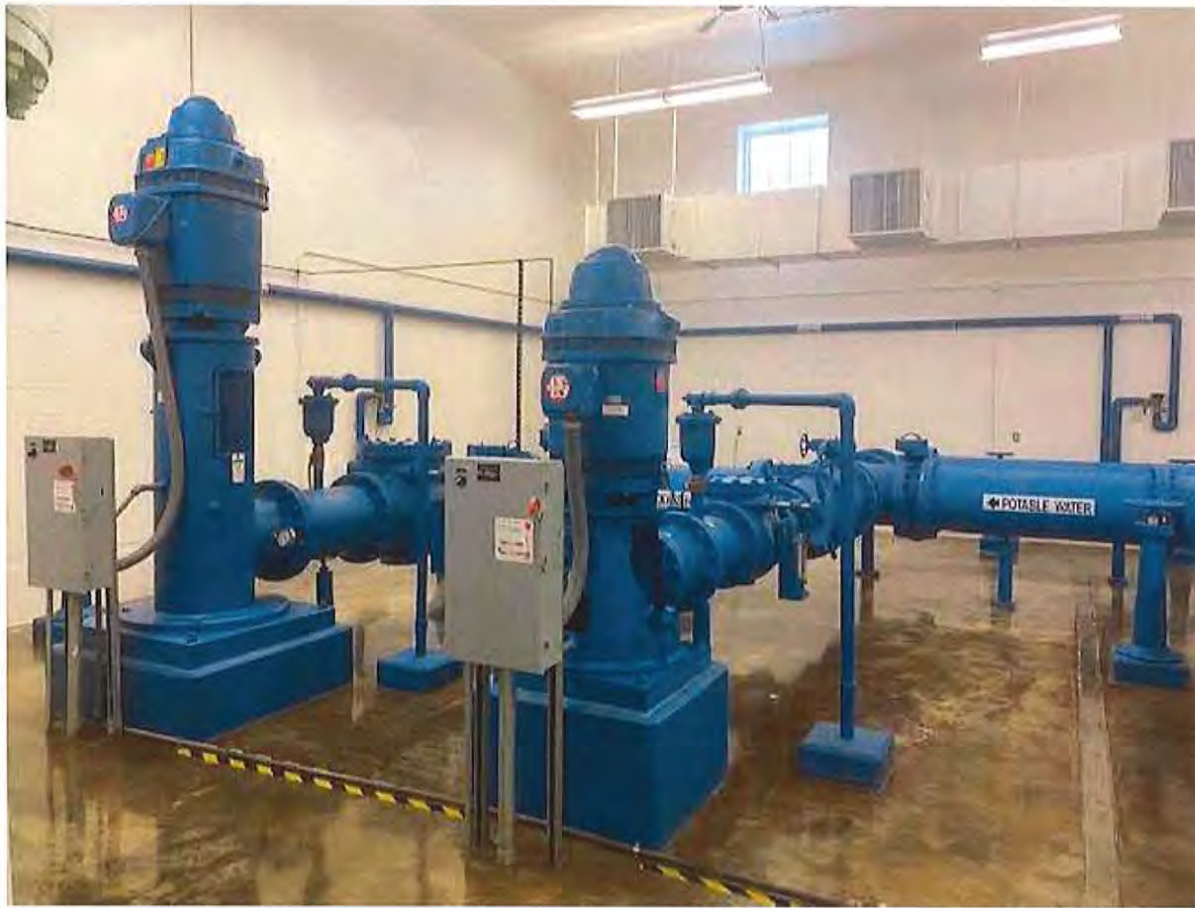
High Service Pump Room
