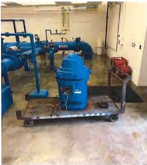
High Service Pump # 2 Motor
