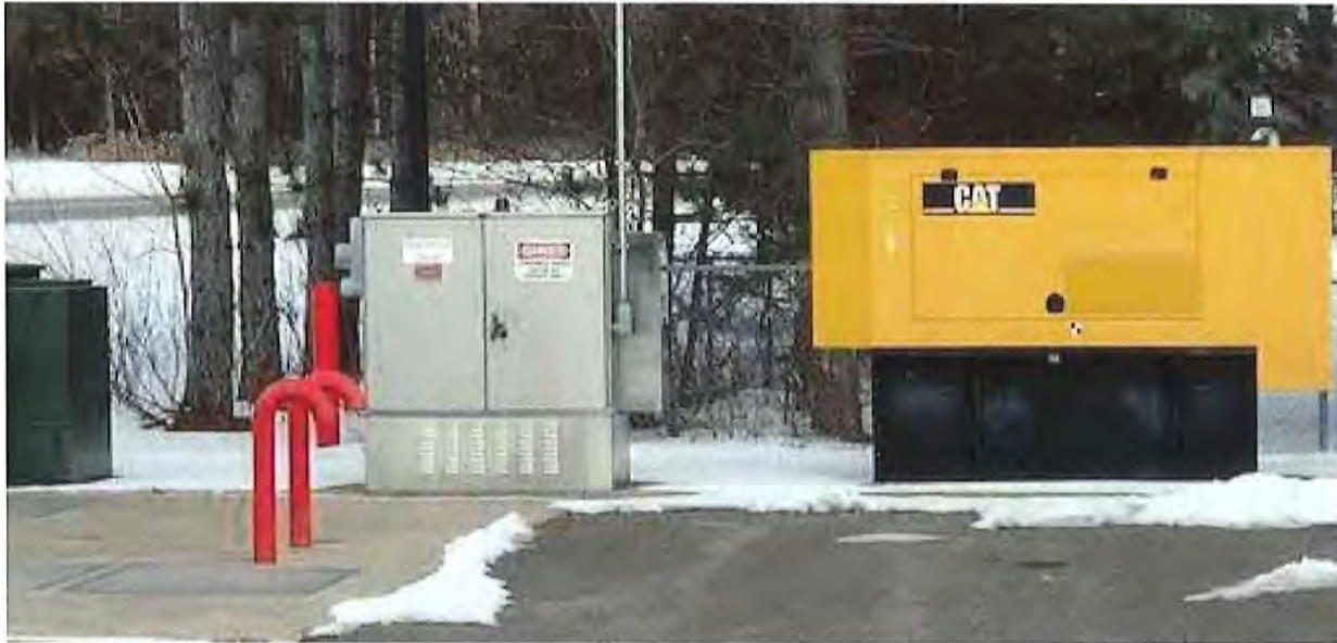
Rivers edge lift station
