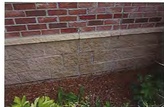
Cracking brick and CMU on west side
